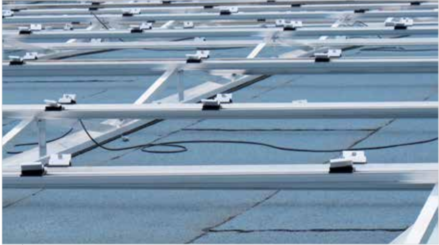
Frankental | Germany System: 58 kW | D-Level System
